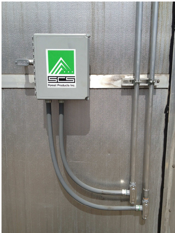
Figure #1 - Hub Box
